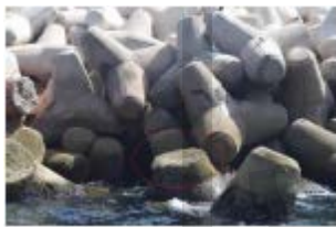
Figure 2. Damages on tetrapods - Breaks and losses
